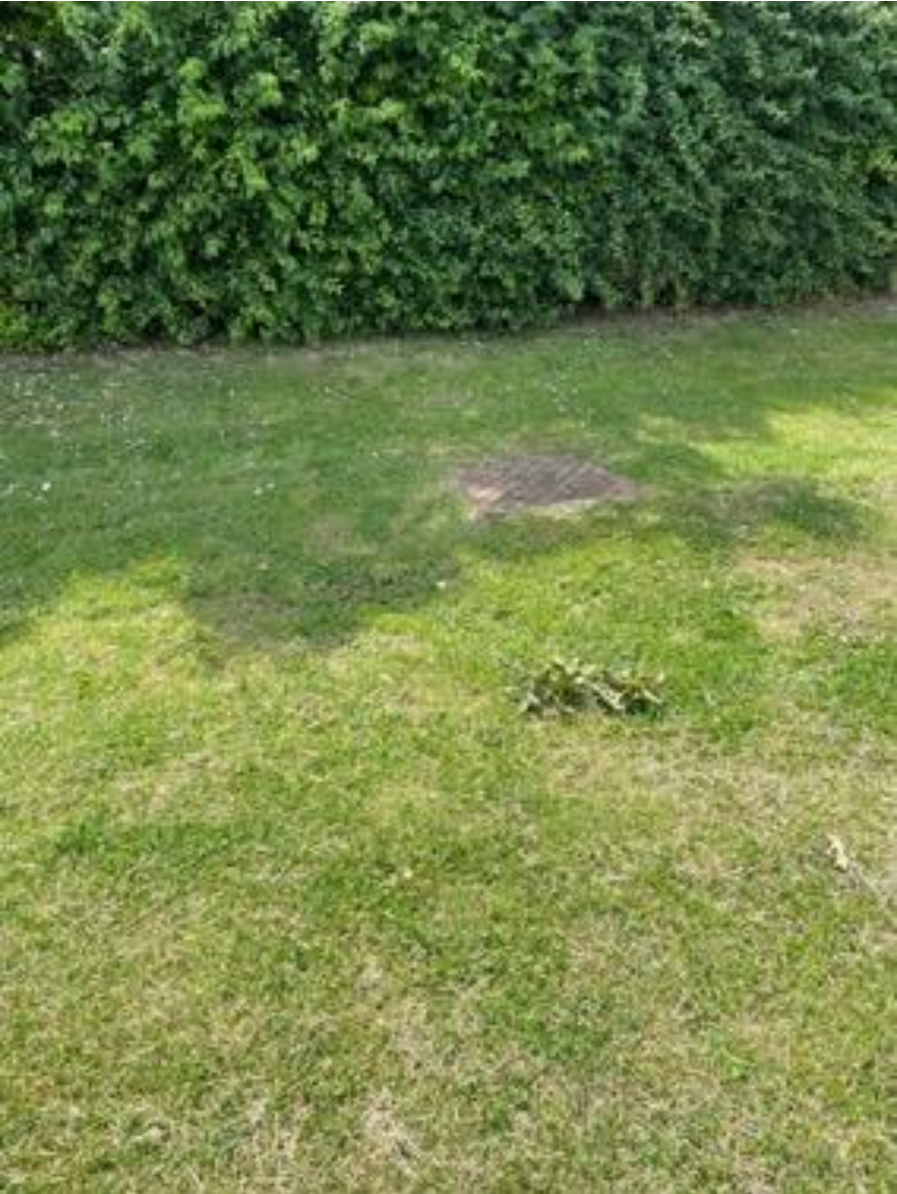
Raised manhole cover
